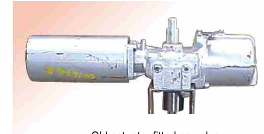
Old actuator fitted on valve
